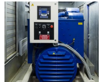
Automatic standby generator
